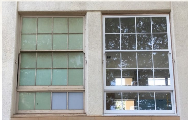
Above: A custom-made wood replacement window (r) prior to painting that is otherwise identical to the original window (l) in operation and materials, including historically-appropriate thin muntins and lugs at the upper sash.
