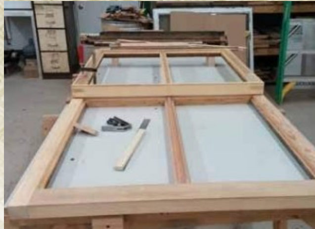
Above: A new, custom-made wood replacement window constructed from a larger salvaged historic window results in a new window out of old growth lumber.
