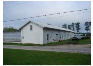
Figure 342. Side view of Greenhouse no. 2.
