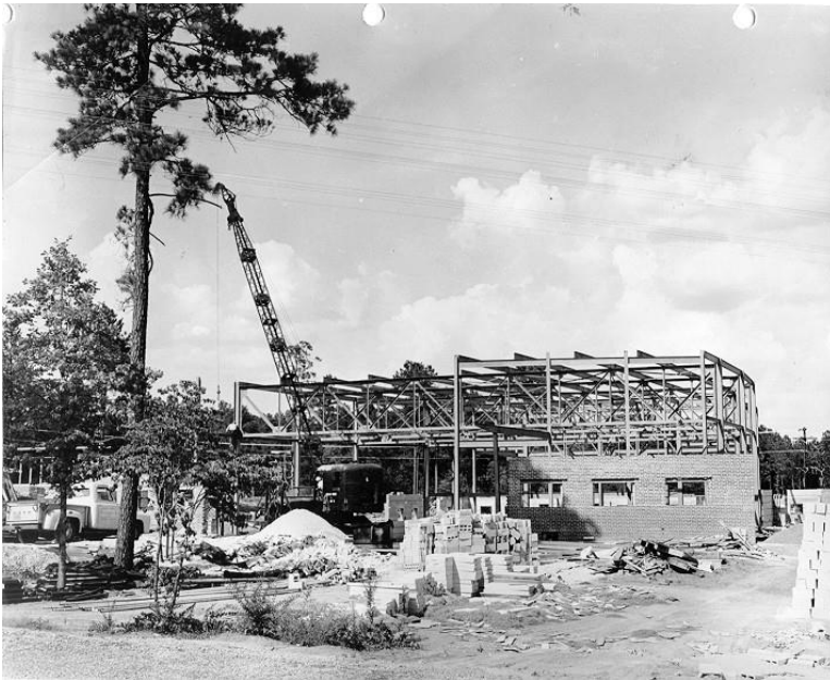
Figure 439. Construction of the Rock Eagle 4-H Center, 1952. (Source: University of Georgia 4-H)
