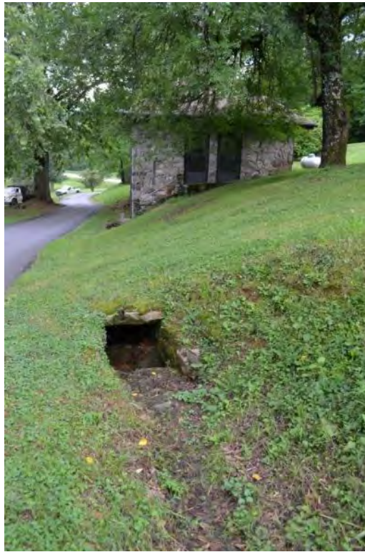
Figure 403. The stormwater management system that parallels Georgia Mountain Experiment Station Road near the Office and Seed Lab.
