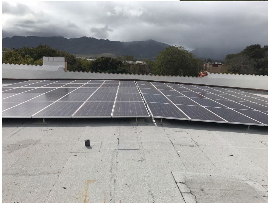
Wheeler Army Airfield Building 104, O'ahu Solar Installation Project, 2017
