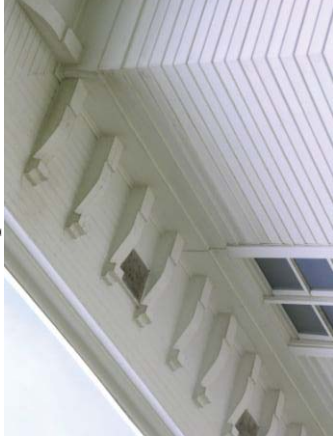
Screened eave vent
