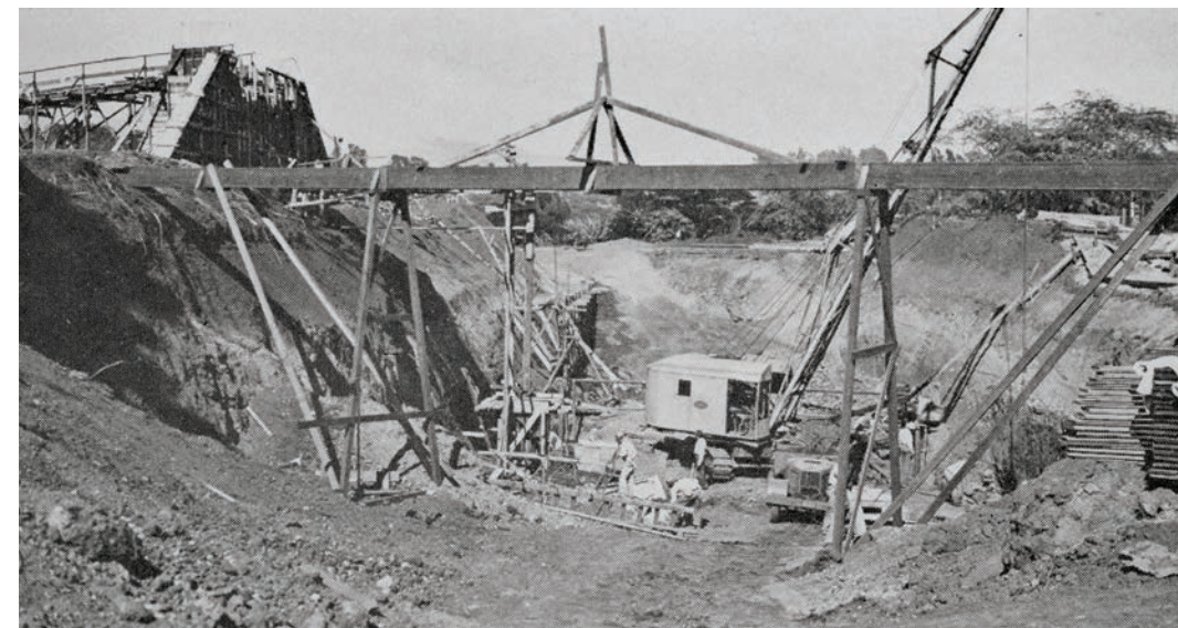
Waialeale Canal Bridge, ca. 1940 Both photos from the Report to the Governor, Territory of Hawai'i, by the Superintendent of Public Works Year ending June 30, 1940
