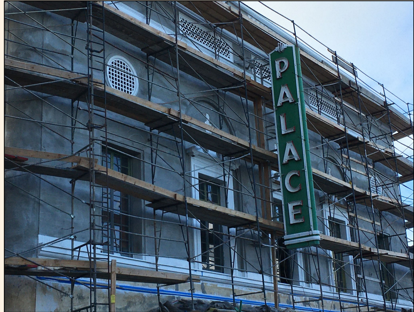
Left: before rehabilitation; Right: stucco application. Photos courtesy of Friends of the Palace Theater
