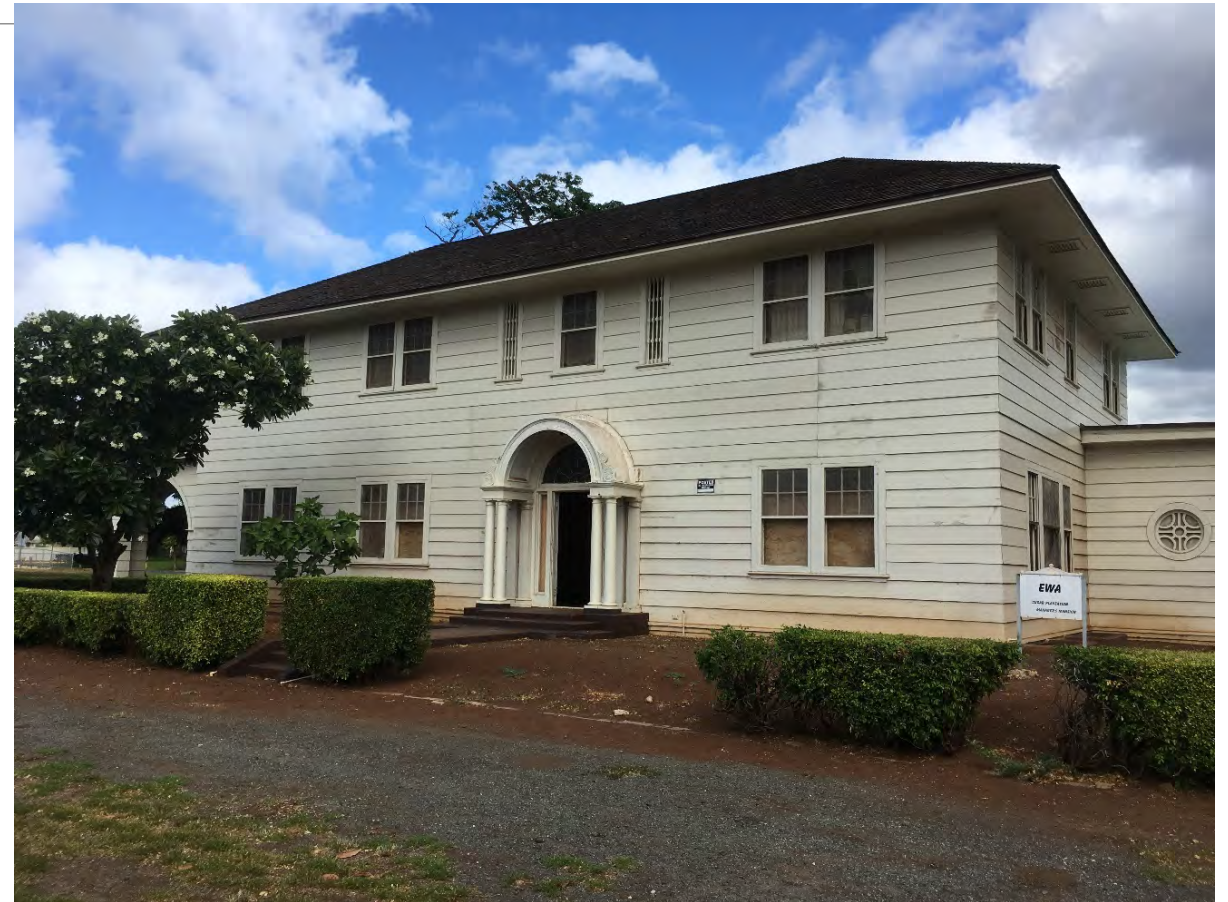
'Ewa Plantation Villages Manager's House is vacant and neglected. Federal funding from Housing and Urban Development grants to the City & County of Honolulu. Photo courtesy MASON
