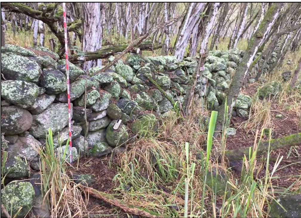
Figure 32. Northern portion of SIHP # 50-80-03-4777 Feature C (intact portion) with periodic areas of collapse about 1 m apart, view to south
