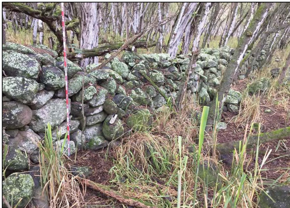
Figure 45. Northern portion of SIHP # 50-80-03-4777 Feature C (intact portion) with periodic areas of collapse about 1 m apart, view to south (Belluomini et al. 2017–draft)
