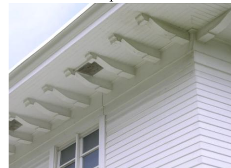
Screened eave vent
