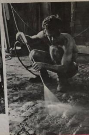
Under a foot of black, oily sand, Tony Hodges found solid red brick. Below, left, Hodges and Boone Morrison construct a new entry.
