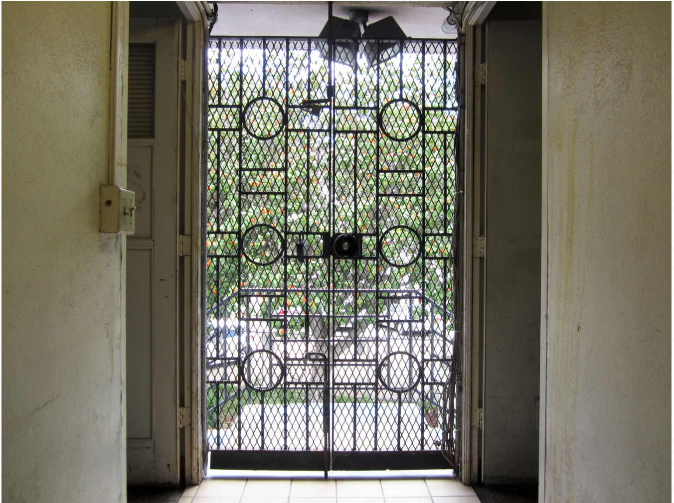
Figure 3: Open entry door detail at south end of second floor hallway. View facing southwest.
