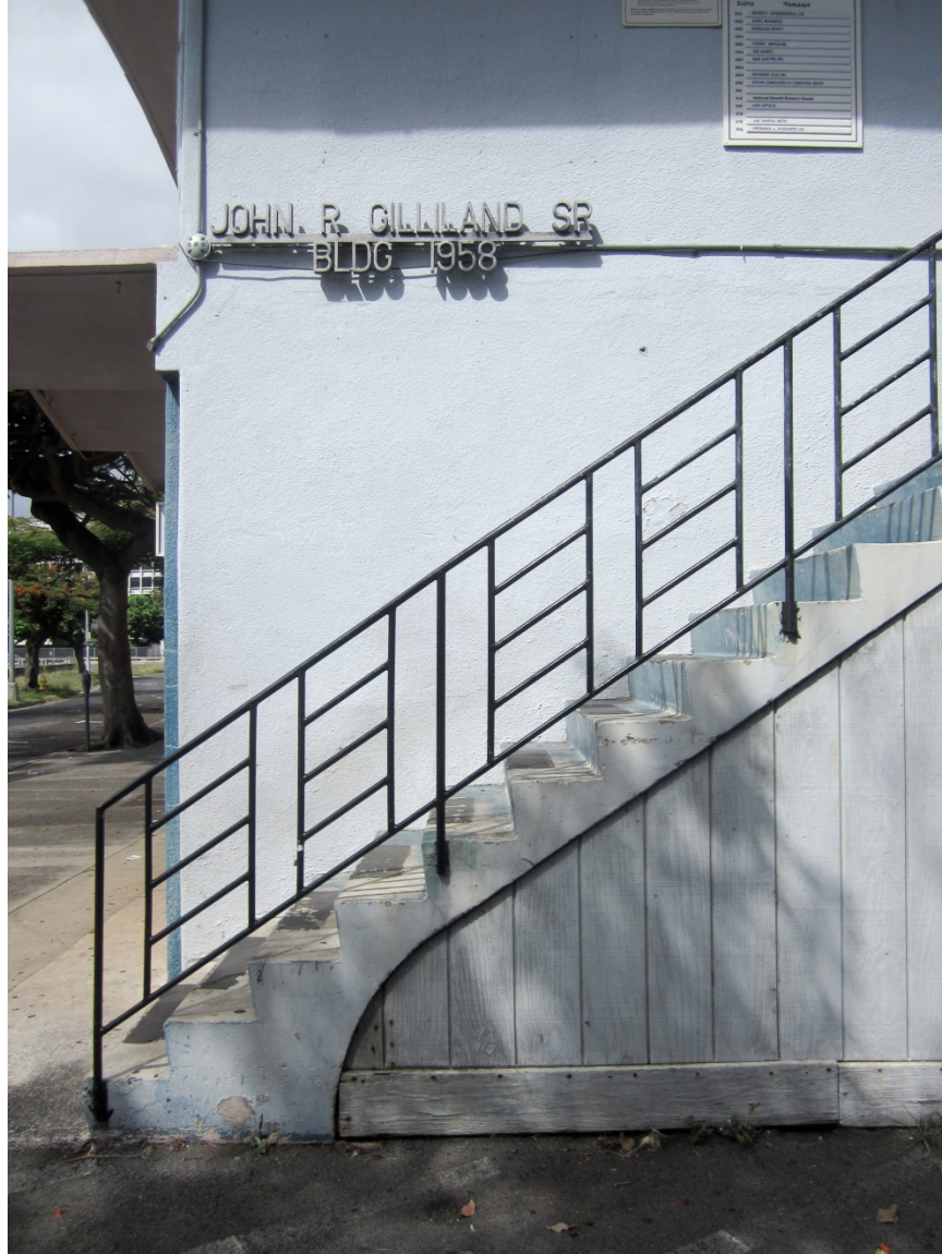
Figure 2: “John R. Gilliland Sr. Building, 1958” nameplate and stair railing detail. View facing northeast.
