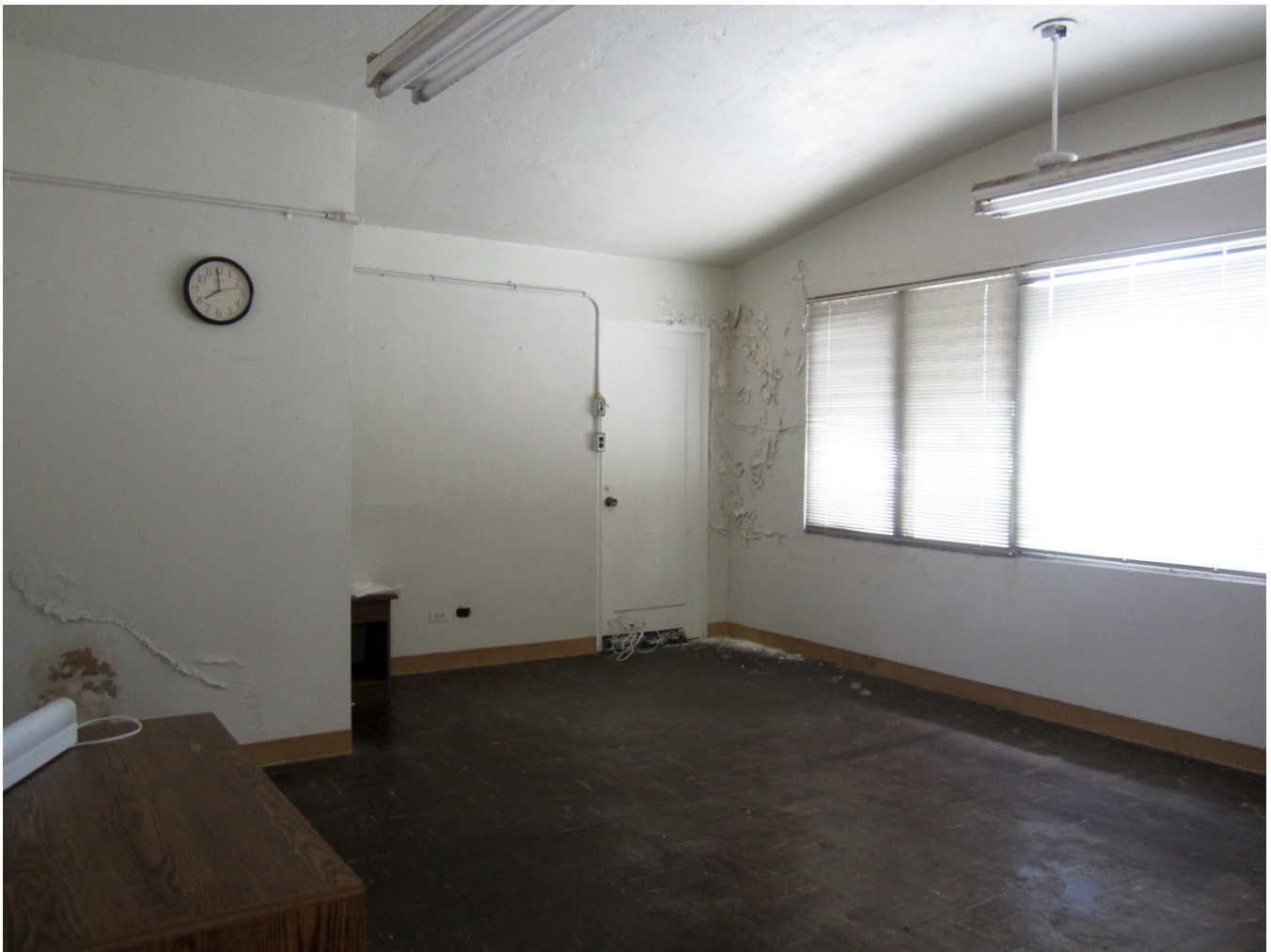
Figure 5: Typical second floor office space with barrel arched roof. View facing east.
