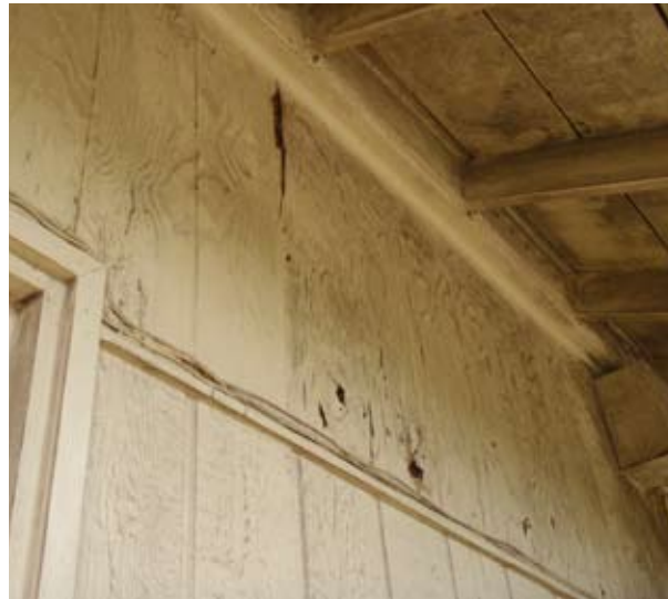
Fig 7.15: Deteriorated Exterior Wooden Wall, 2008
