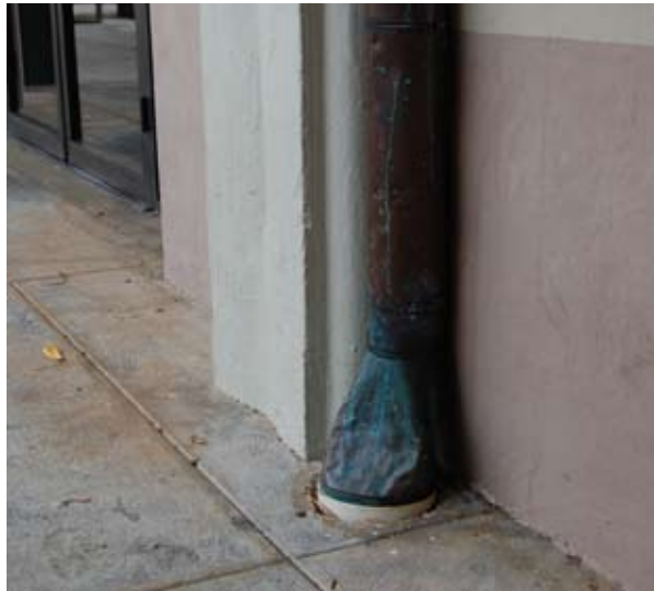
Fig 7.18: Deformed Metal Drainpipe at Hemenway, 2008
