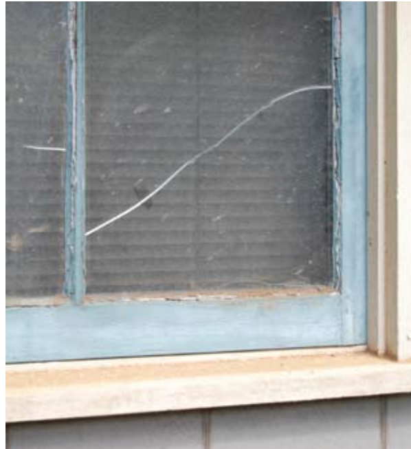
Fig 7.27: Cracked window detail at Krauss Hall Annex, 2008
