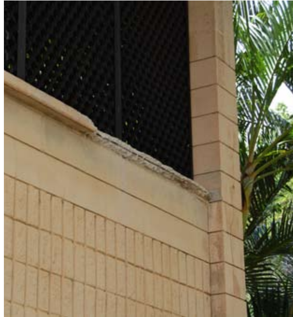
Fig 7.5 Damaged Masonry Ledge at Hawaiian Institute of Geographics, 2008
