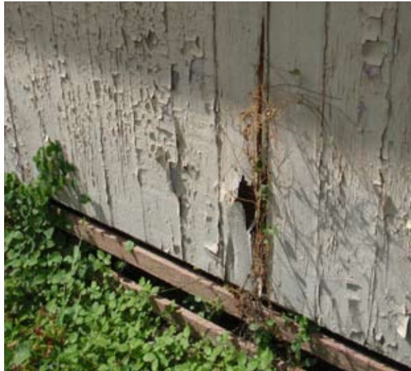
Fig 7.16: Deteriorated Exterior Wall at University High School, 2008
