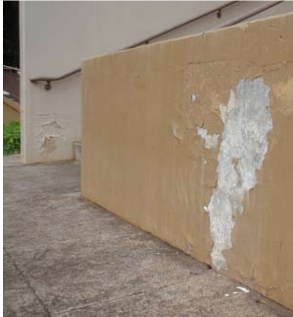
Fig 7.35: Water Damage on Exterior Walls, 2008
