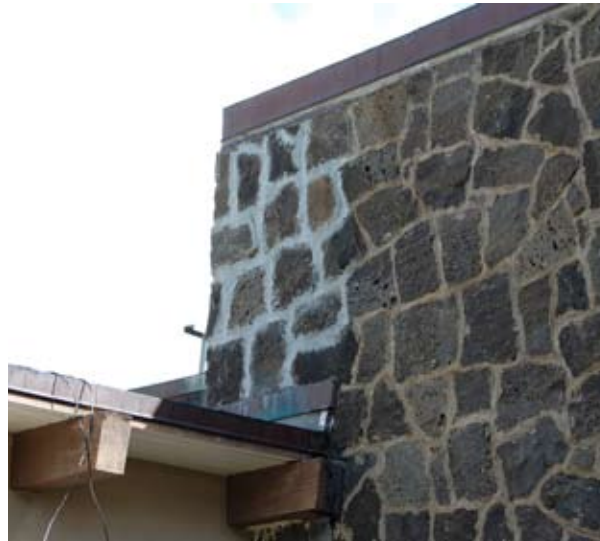
Fig 7.6: Mismatched Color and Mortar Size at the Administrative Services Building, 2008
