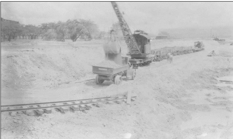
Figure 54. A locomotive crane removes and loads fill from a coral pit for repairs to North Road. 27 April 1928. Hawaiian Railway Society.
