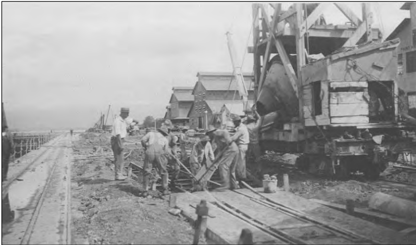
Figure 44. A concrete mixer atop a flatcar assists in the paving of concrete and trackage around the Dry Dock, 20 January 1921. Hawaiian Railway Society.
