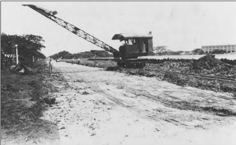
Figure 53. A locomotive crane assisting in the repaving of Avenue E and the driveway to the Administration Building, 4 April 1927. Hawaiian Railway Society Collection.
