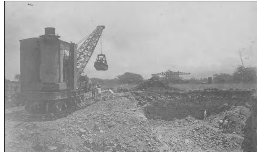
Figure 35. Locomotive crane involved in excavation of a water reservoir, north of Fac. 1, 3 July 1918. Hawaiian Railway Society Collection.
