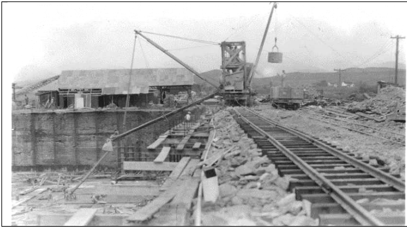
Figure 34. A flatcar of concrete supplies a concrete mixer (also atop a flatcar) for Fuel Oil tank construction, 30 April 1919. Hawaiian Railway Society Collection.
