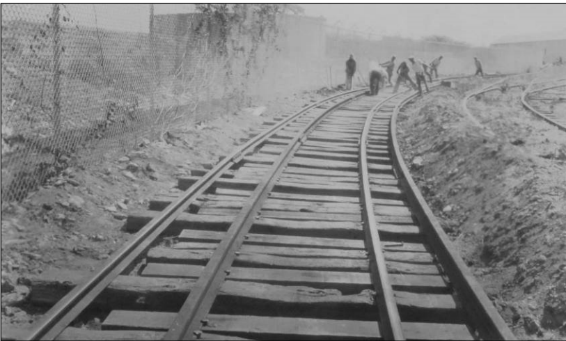
Figure 58. Navy Yard laborers work to replace 1,216 feet of track leading to the West Gate. View looking southwest. Record Group 71, National Archives and Records Administration.
