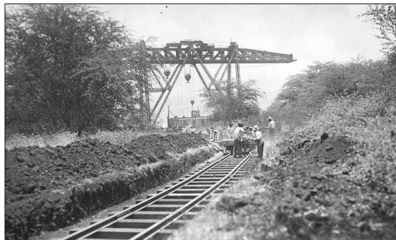
Figure 37. Yard laborers completing railroad work toward the Torpedo Boat Piers. View looking northeast, 5 July 1918. Record Group 71, National Archives and Records Administration.
