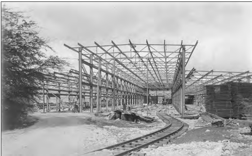
Figure 48. Railroad trackage involved in the construction of a new storehouse (Building 68), 10 January 1923. Record Group 71, National Archives and Records Administration.
