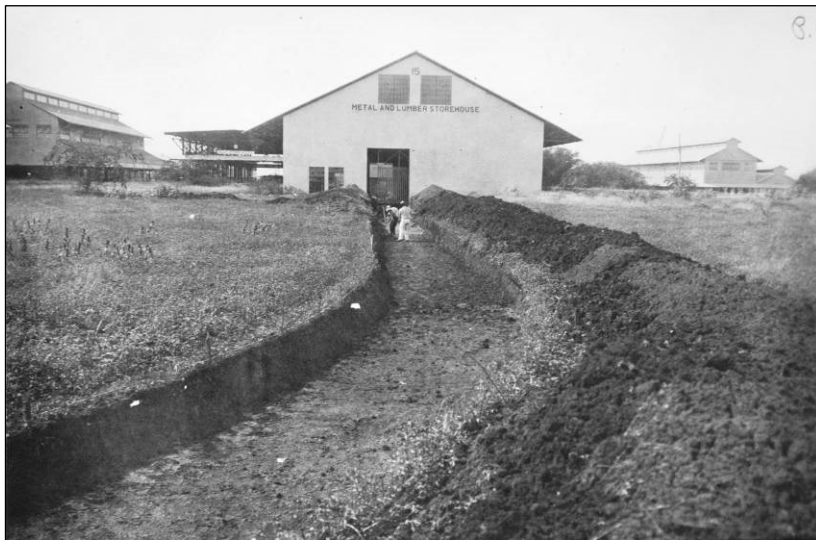
Figure 31. Preparation of railroad bed into Fac. 15, Metal and Lumber Storehouse, March 1916, view looking northwest. Record Group 71, NARA.
