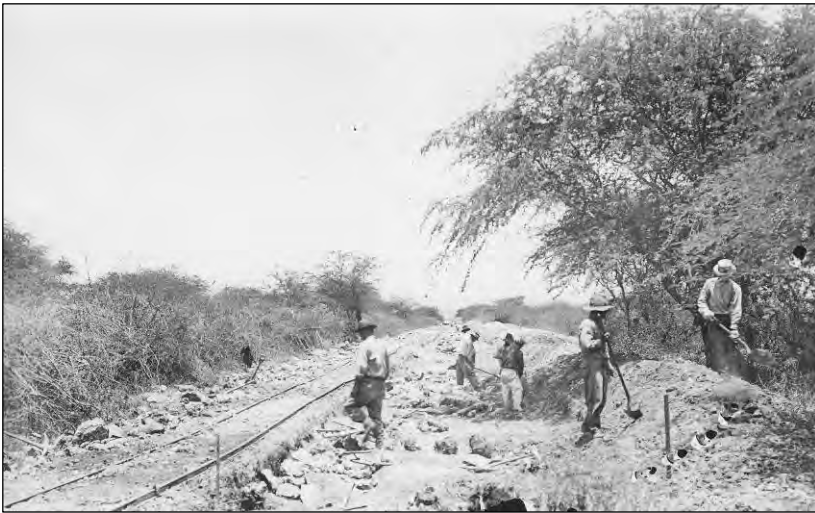
Figure 42. The railroad spur to Watertown that lead out of the Navy Yard's southwestern gate, August 1916. Photo taken near where the railroad crossed South Avenue. Record Group 71, National Archives and Records Administration.
