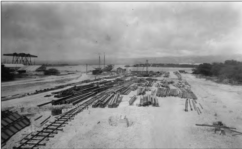
Figure 47. Railroad involvement in site preparation for the construction of a storehouse (Building 68), 24 May 1922. Record Group 71, National Archives and Records Administration.
