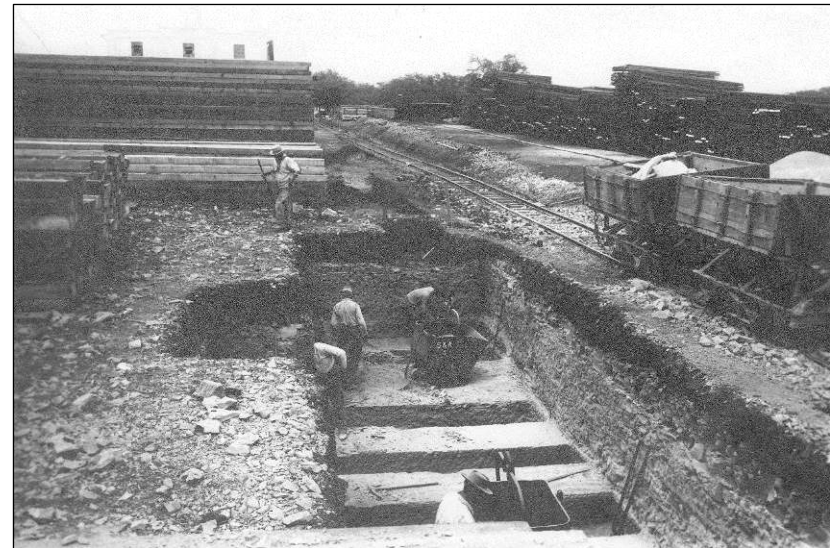
Figure 32. Construction of the railroad track scale located along Avenue D (what is today Paul Hamilton Avenue), April 1915. Record Group 71, NARA.
