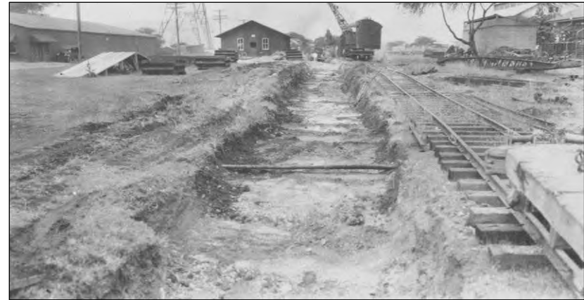
Figure 55. A locomotive crane assists in the excavation of foundation for new trackage. View taken from Second Street looking west, 3 May 1928. Hawaiian Railway Society Collection.
