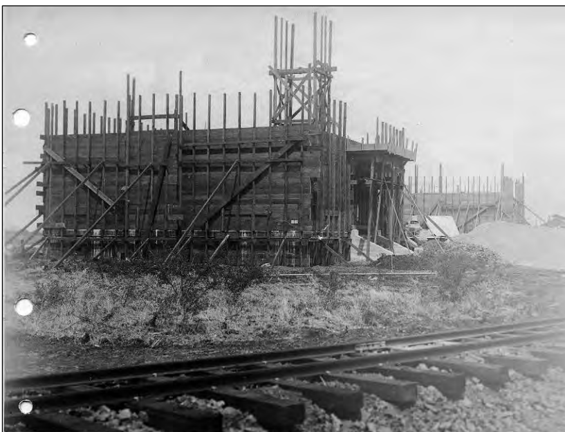
Figure 18. View of construction of three Officers Quarters for the US Marine Corps at the Naval Station, 4 August 1912 (left to right: Fac. 201, 202, and 203). The permanent trackage in the foreground was the line that paralleled Central Avenue. Library of the Marine Corps.
