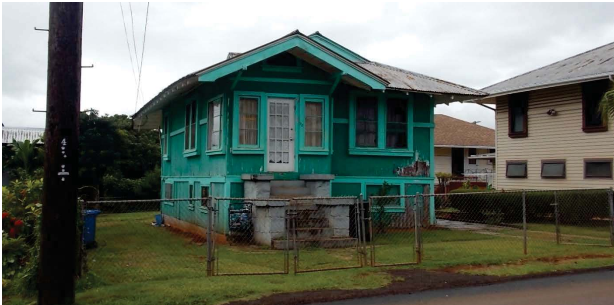
75 Kuahiwi Avenue, built in 1934, is representative of the types of residences that may be a good candidate for a National Register listing under an MPD.
