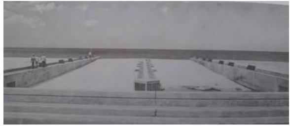
4-101 Ulehawa Stream Channel Outlet Structure Features a Unique Design of By-pass (City and County of Honolulu Public Works Annual Report)
