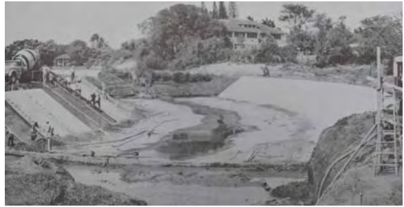
4-102 Kaupuni Stream Channel Construction (City and County of Honolulu Public Works Annual Report)
